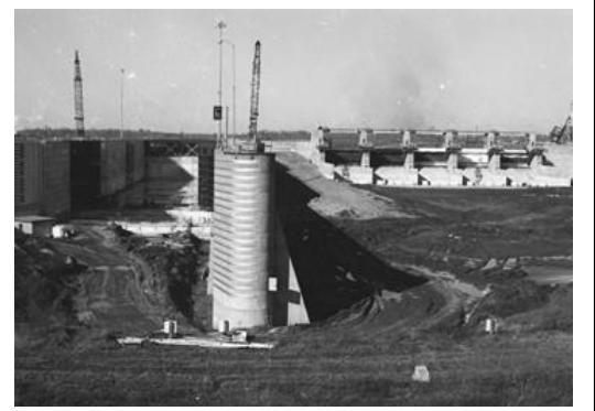
Picture of Columbus Lock and Dam under construction behind where the Plymouth Bluff Environmental Education Center is today. Taken from below the dam which is in the river bed today. Photo by J. Guyton 1978.
